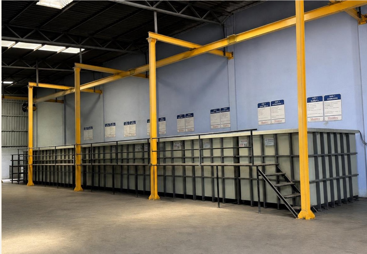
8-Tank Pretreatment System
